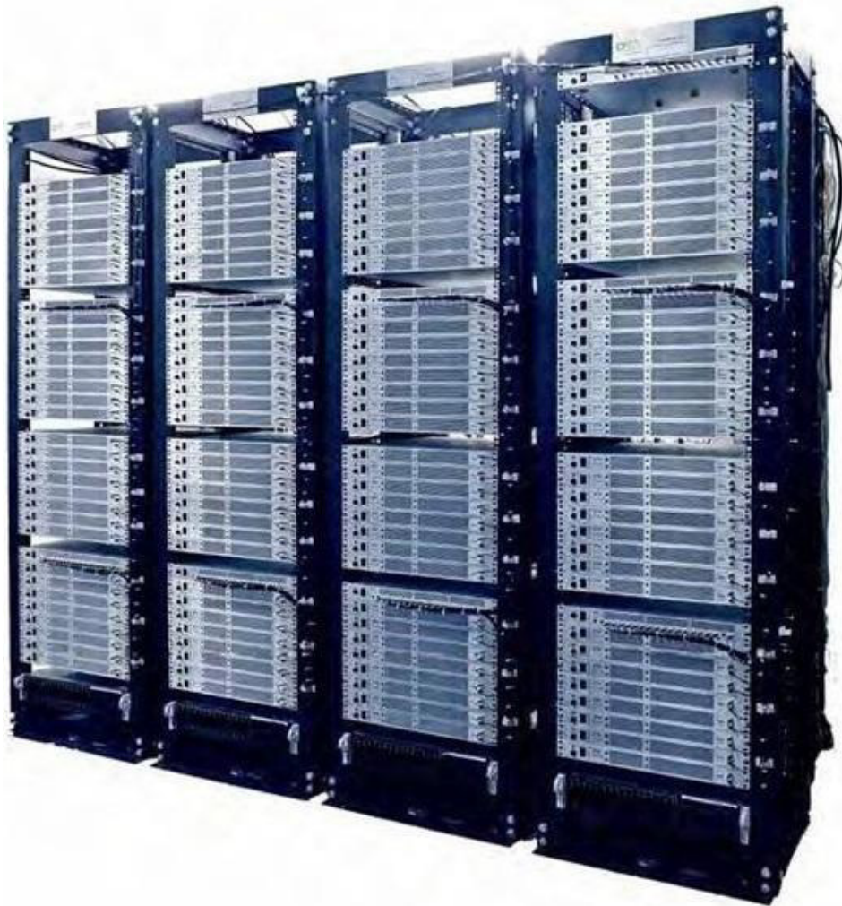
Figure 1: 1024 receive channels are distributed across 4 identical racks with 256 channels in each rack. All 1024 channels operate synchronously across 4 racks with less than 1ns timing skew.
