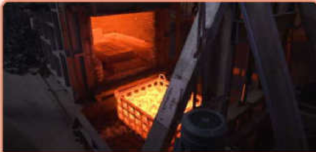
Heat Treatment Furnace
