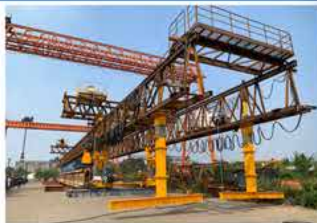
▶ FACTORY TESTING YARD
