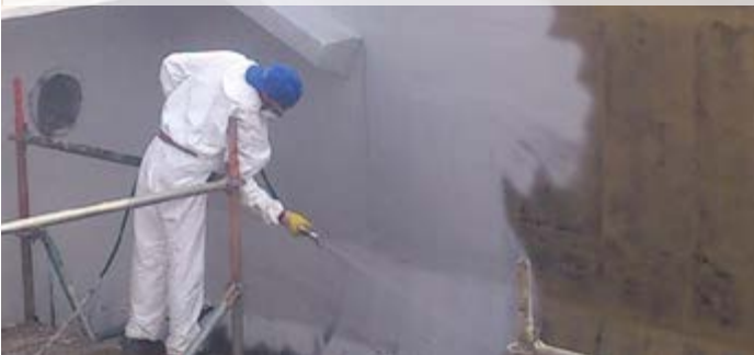
► Refurbishment of a buffer tank in a sewage plant – available only in English language
