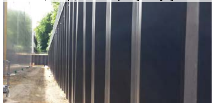
► Durable corrosion protection and weathering resistance for sheet pile construction (1.800 sqm) – available only in English language
