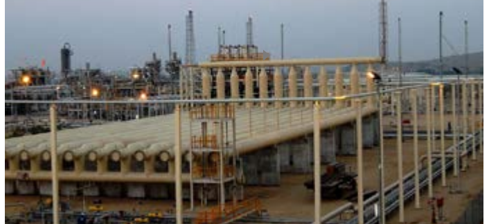
► Internal coating of slug catcher pipelines for the extraction of natural gas – available only in English language
