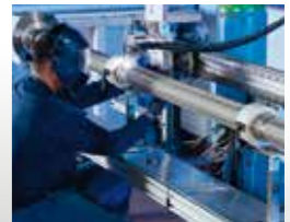
PACO employs welding systems designed and built by the in-house mechanical engineering team for the production of its filters – for example, to produce extremely long filter elements (up to 4.200 mm).
