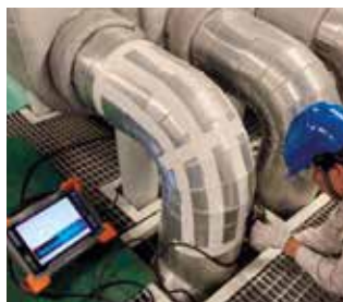
Corrosion under insulation (CUI)
