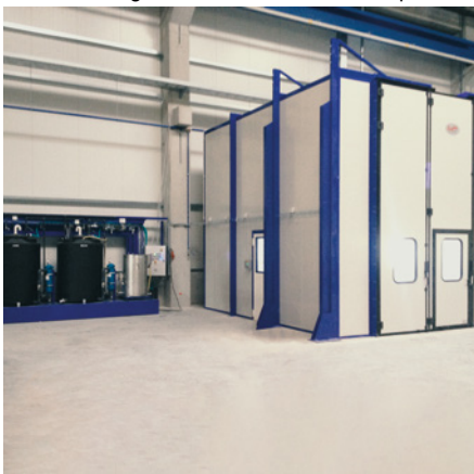
➤ Closed cycle liquid recovery skid
